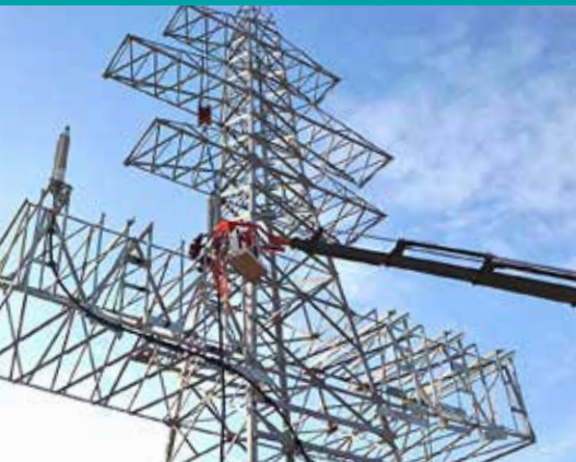
Lifting 170 kV dry type outdoor termination with no need for scaffold on tower.
